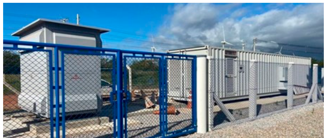
Figure 7. BESS installed on CDV.
