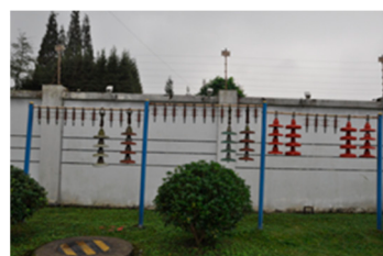
Figure 12. The CBS substation site testing point.
