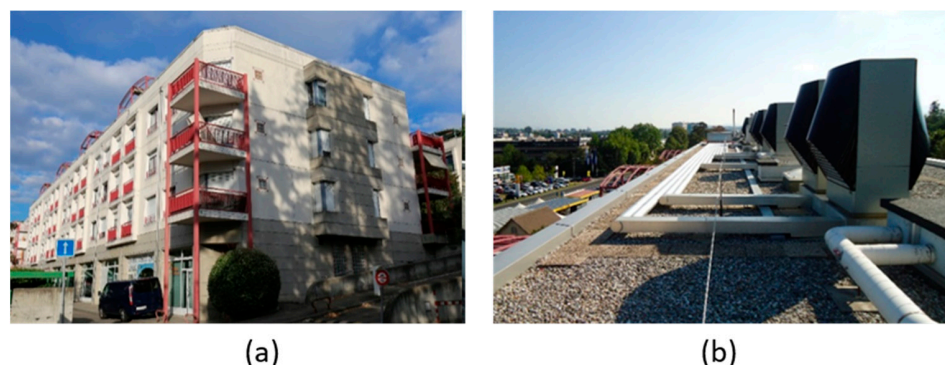
Figure 4. Hybrid ASHP system. (a) Non-retrofitted MFB and (b) six air-to-water heat pumps on the roof.
