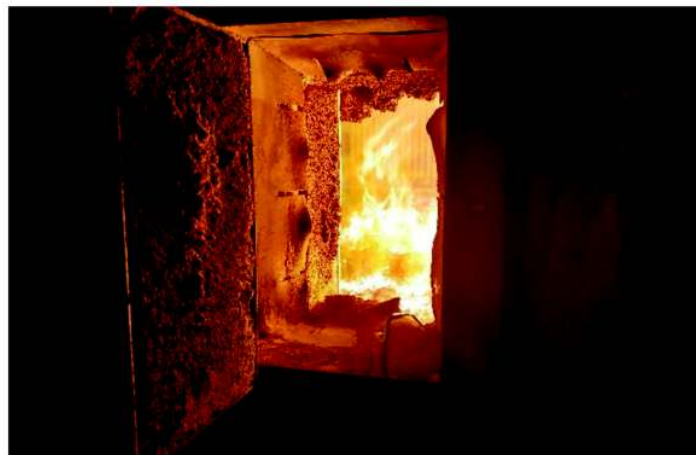
Figure 4. The middle part of grate—view from the middle inspection door of the boiler.
