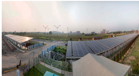
Figure 7. Bird's eye view of the 500 kWp canal top solar PV power plant installed at Newtown, Kolkata.
