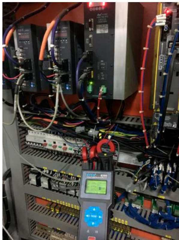
Figure 7. Grinding machine current monitor.
