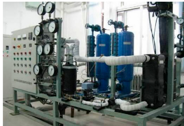
Figure 5. The test-bed of a compression refrigeration system.
