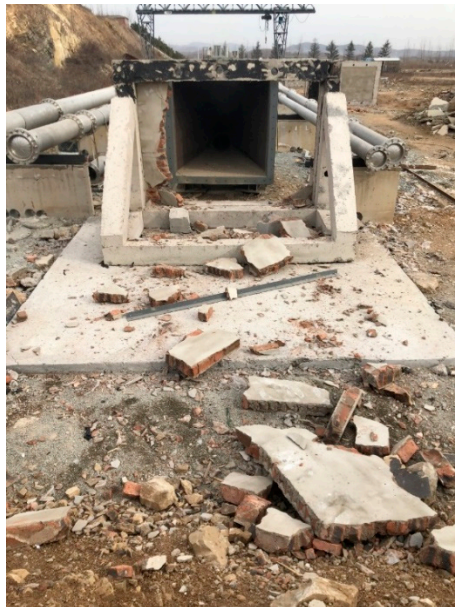
Figure 10. Distribution of debris after the failure of the unstrengthened wall.
