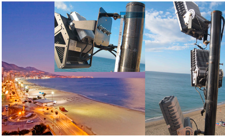
Figure 1. Overview of the study lighting installation area and evidence and detail of two models of LED projector mounted on our test pole.
