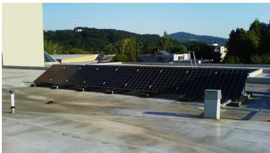
Figure 6. Photovoltaic (PV) panels.
