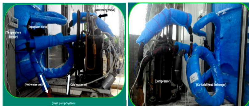
Figure 5. Installed heat pump systems with a co-axial heat exchanger.
