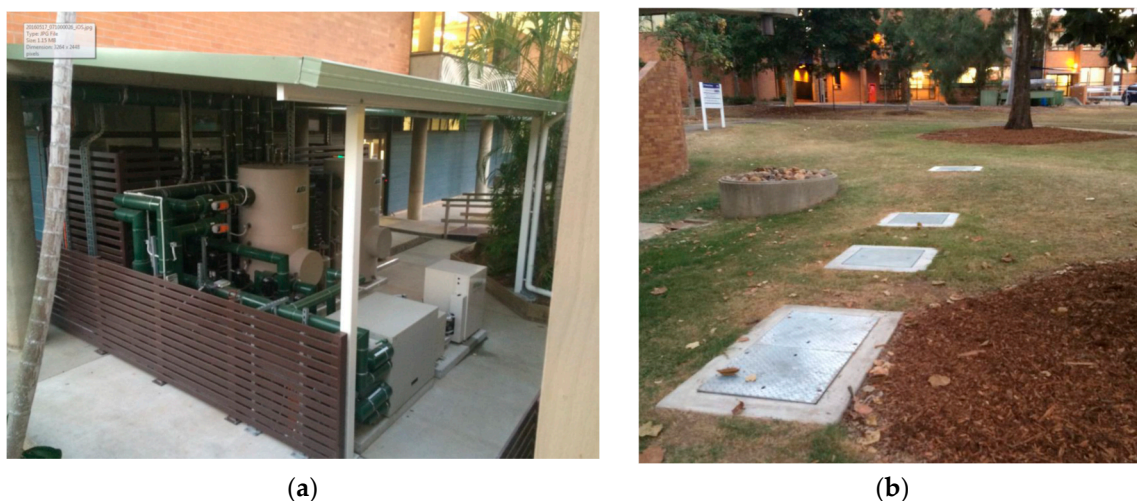
Figure 1. (a) The main ground components of the ground source heat pump (GSHP) system; and (b) the three monitoring wells in direct expansion (DX) loop.
