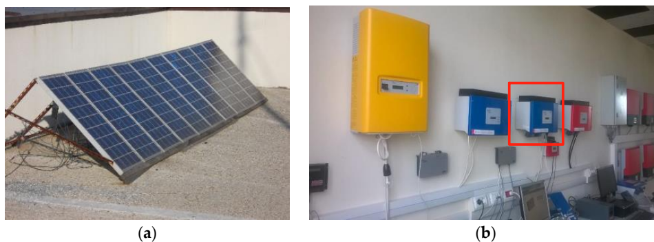
Figure 4. The components of the subsystem 1: (a) 10 photovoltaic panels; and (b) the Sunny Boy SB2100TL inverter.
