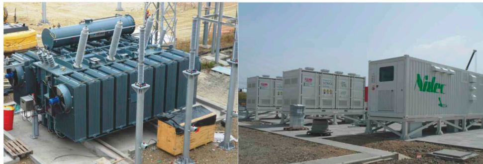
Figure 5. Some photos of the Italian “power intensive” installation (Storage Lab) in Codrongianos.
