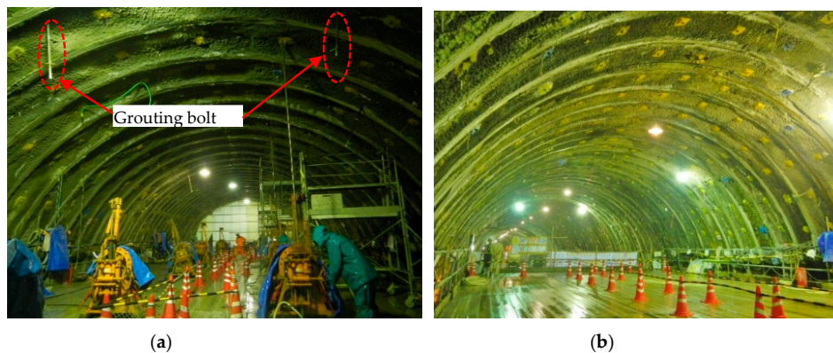
Figure 17. The effect of the new grouting method. (a) The grouting process; (b) the effect after grouting.
