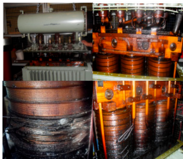
Figure 12. Visual inspection showing deformation of winding (W) [21].
