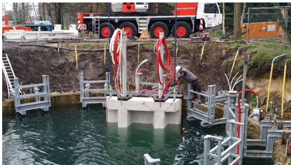
Figure 1. Construction of an Ecovat buffer in Uden, the Netherlands [18]. This Ecovat buffer is 16 meter deep with a diameter of 11 meter. However, in the future construction of even larger buffers is planned.
