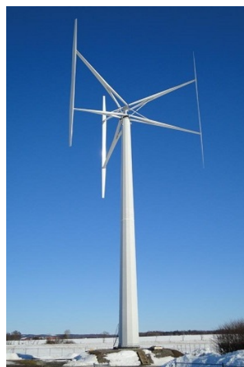
Figure 2. The three bladed 200 kW vertical axis wind turbine in Falkenberg, Sweden.
