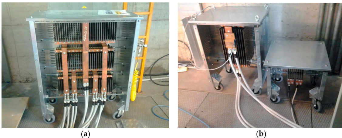
Figure 10. (a) Dummy load for the cathode power supply (6 star-connected resistors); (b) Dummy loads for the pinch (on the left) and PFC power supplies with their measurement shunts.
