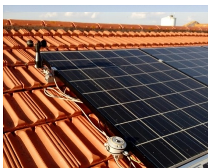
Figure 5. Pyranometer and anemometer installed on the roof.
