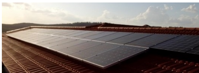
Figure 2. Roof mounted PV system.
