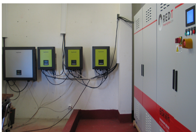
Figure 3. VRFB (right) and the inverters (left).
