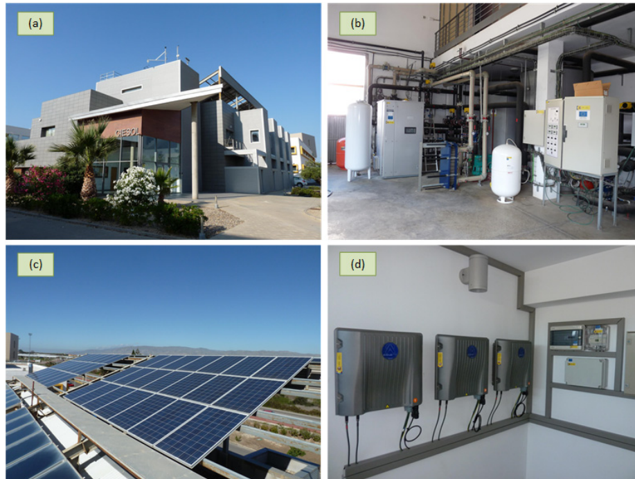
Figure 1. The Solar Energy Research Center (CIESOL or Centro de Investigación en Energía SOLar in Spanish) building: (a) exterior of the CIESOL building; (b) solar cooling installation; (c) photovoltaic (PV) power plant: PV panels; and (d) PV power plant: PV inverters.
