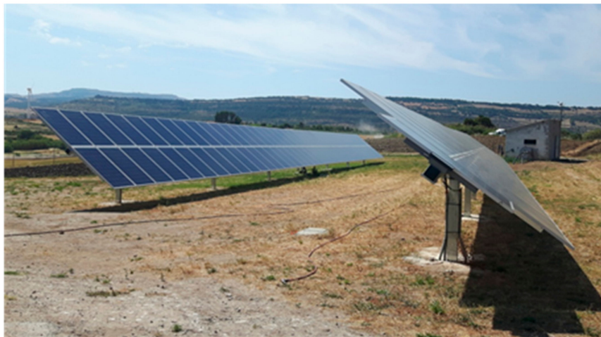
Figure 3. Stand-alone PVIS installed in Uri (Sassari, Italy).
