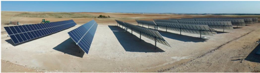
Figure 2. Stand-alone PV irrigation system (PVIS) installed in Alaejos (Spain).
