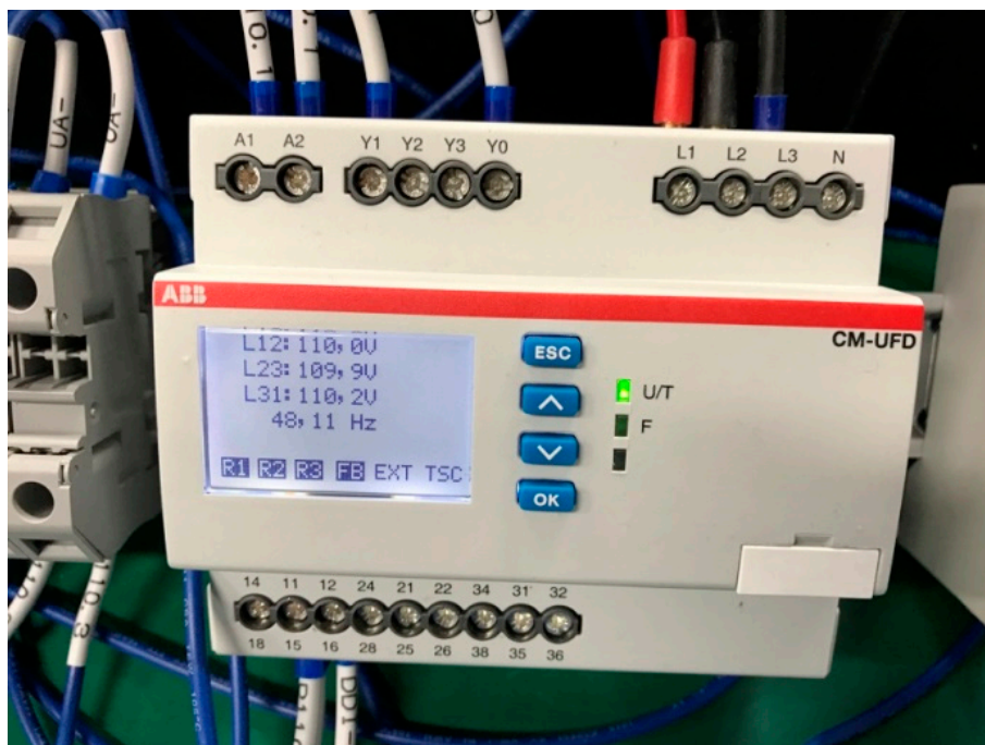
Figure 31. Resetting under frequency relay.
