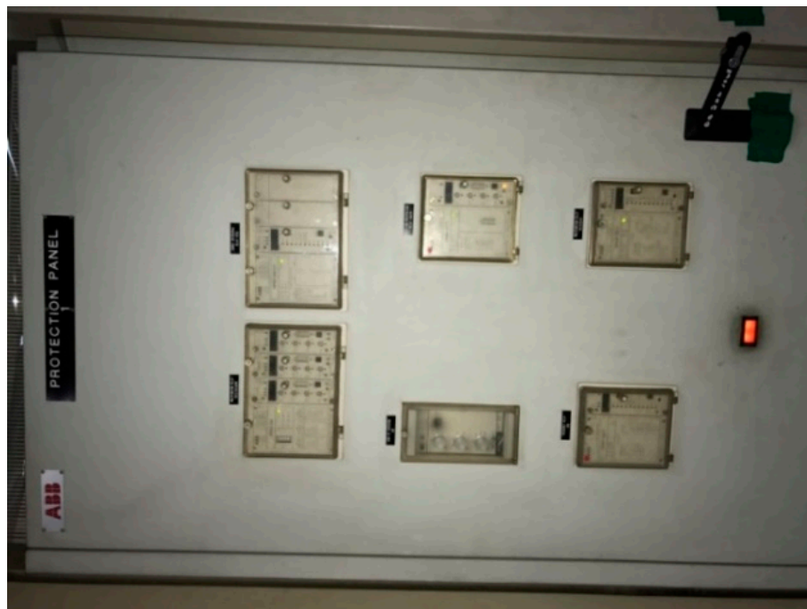
Figure 34. Operation of protection panel.
