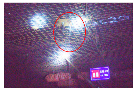
(f) The bolts water
