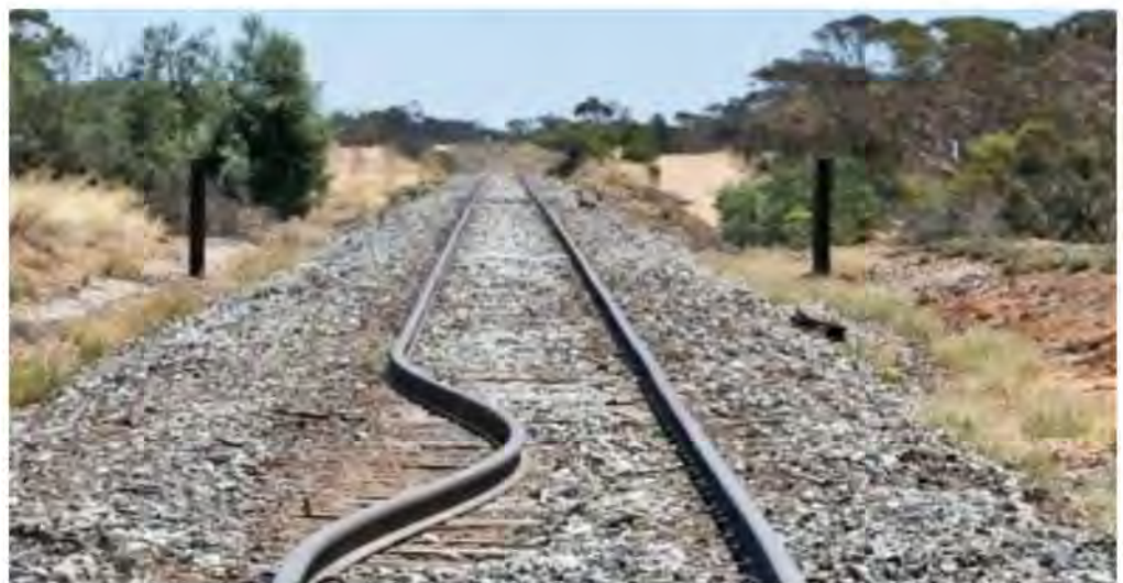
Figure 2. Track buckling due to high temperatures (source: [7]).
