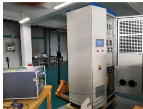
(a) Power Electronic Converter and Tap Switches
