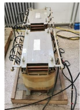
(b) Main Transformer
