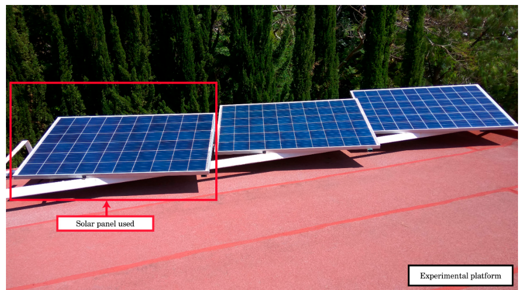
Figure 16. Eco Green Energy EGE-260P-60 solar panel used.
